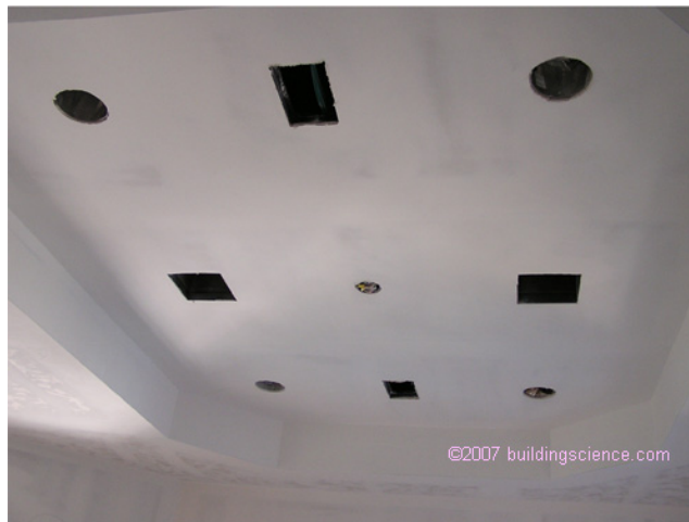
Photograph 1: Ceiling Penetrations – “Swiss Cheese Services”
